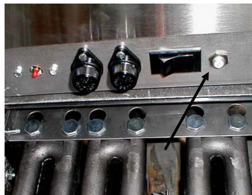
A resettable circuit breaker protects the filter circuit.
